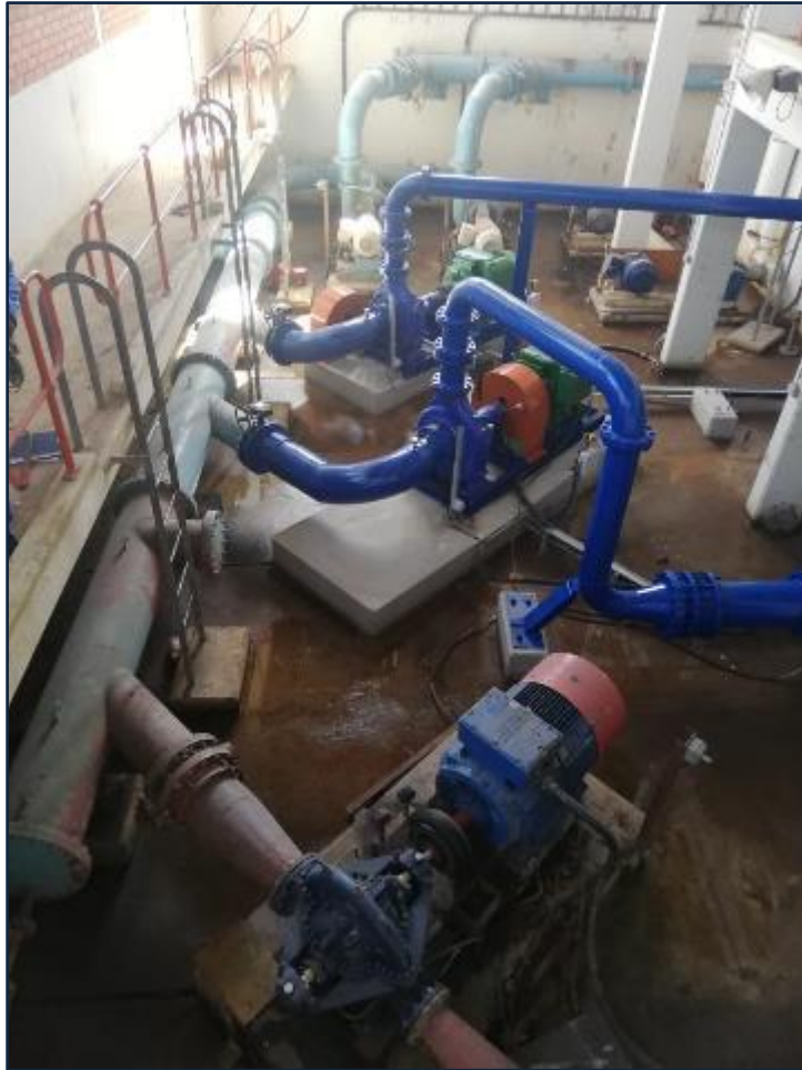
Figure 13.42 Olifantskop Clear Water Pump Station (Umgeni Water 2019).
