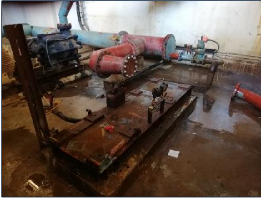
Figure 13.46 Petronella pump as of May 2019 (Umgeni Water 2019).
