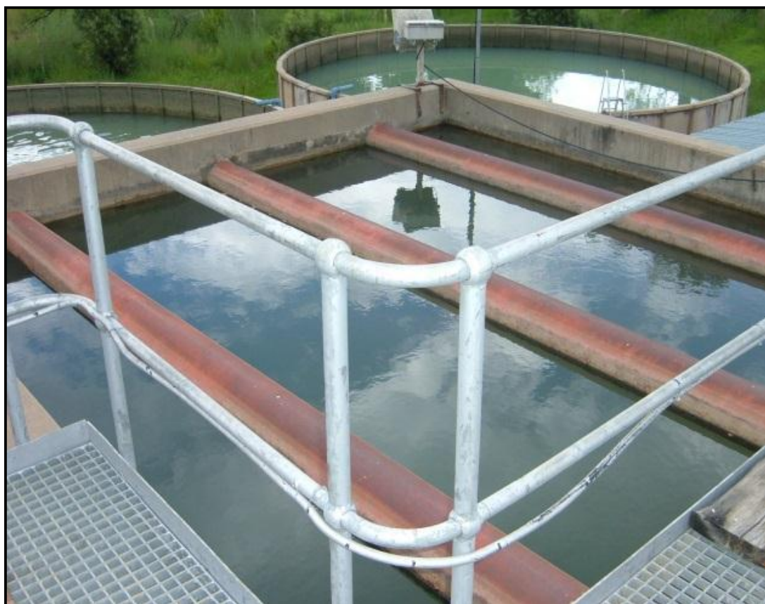
Figure 13.55 Colenso WTP (Umgeni Water 2017)
