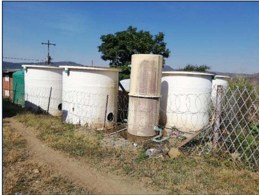
Figure 13.33 Tugela Estates WTP clarifiers (Umgeni Water 2019).
