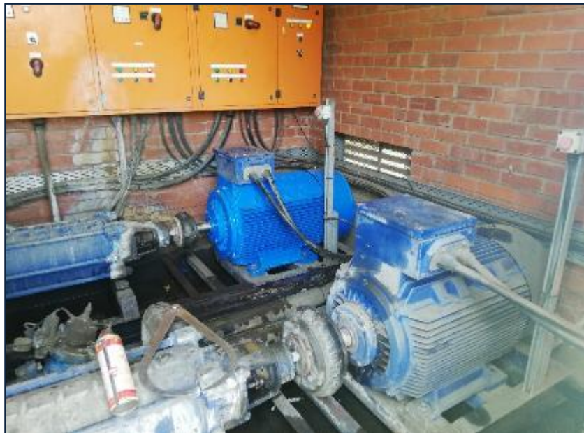
Figure 13.28 uMhlumayo Pump Station (Umgeni Water 2019).
