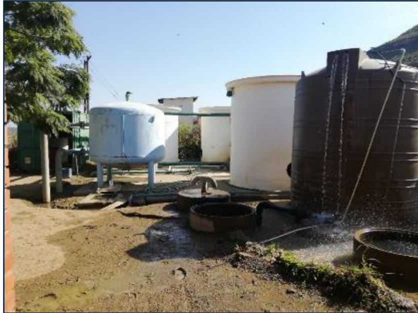
Figure 13.27 Tugela Estates Water Treatment Plant (Umgeni Water 2019).
