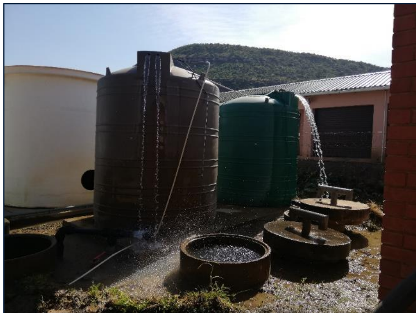
Figure 13.34 Tugela Estates WTP reservoirs (Umgeni Water 2019).
