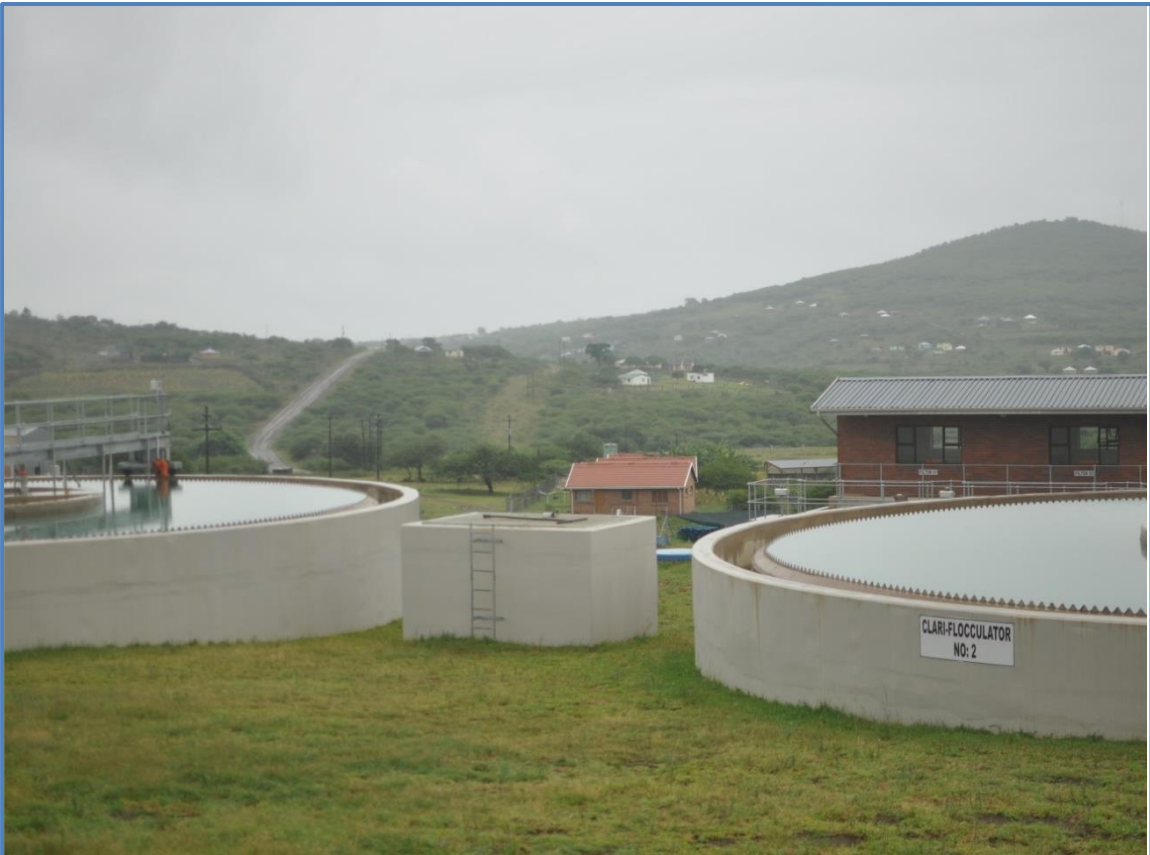
Figure 16.14 Photo of Middledrift WTP Clarifiers.
