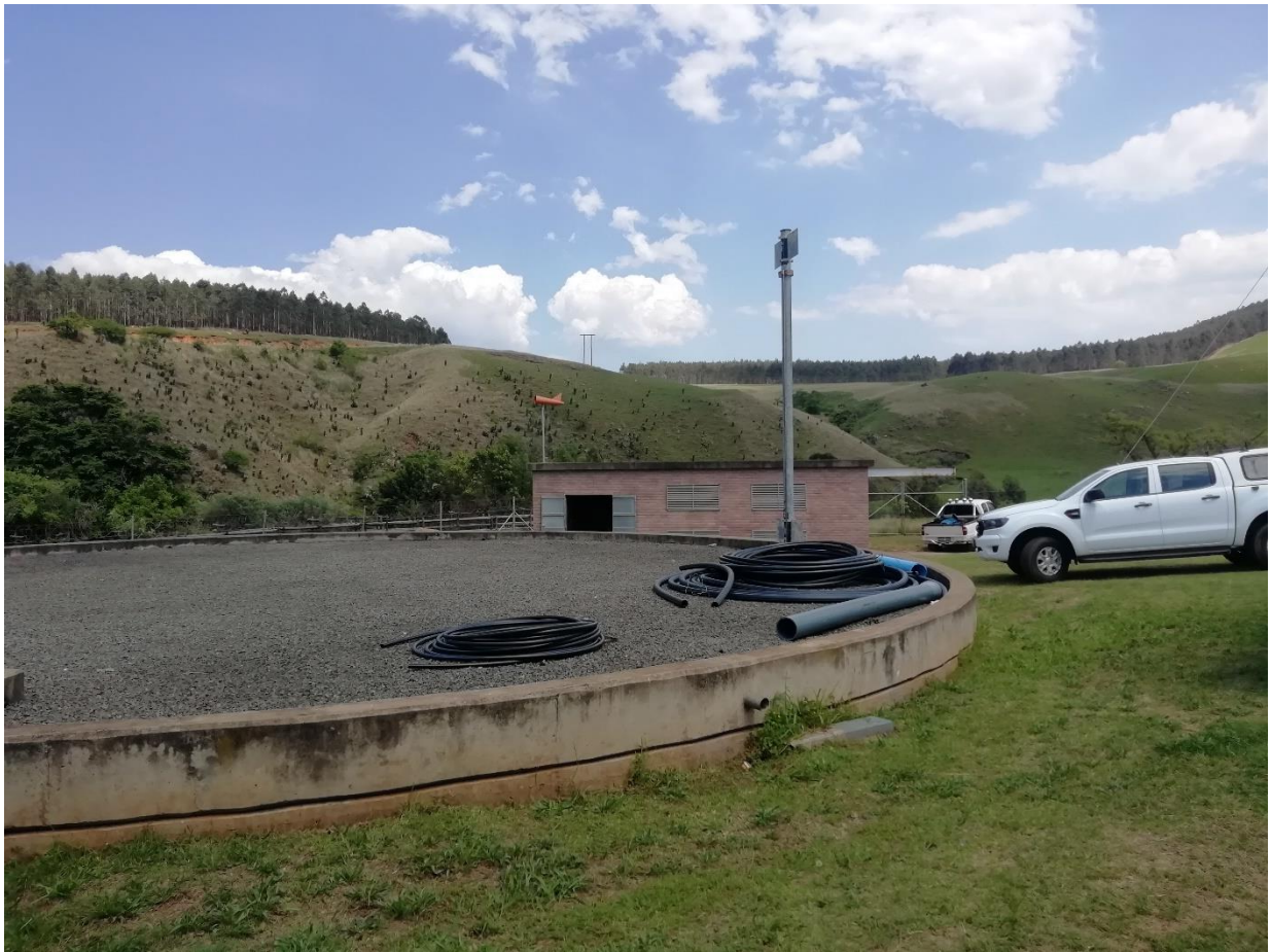
Figure 16.10: The Nkandla WTP (Photo taken by UW).
