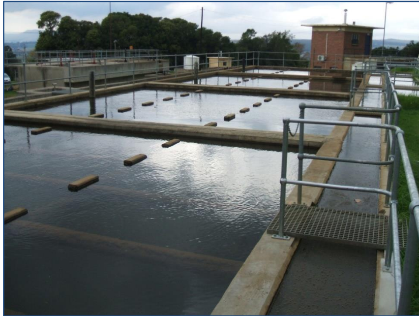
Figure 7.84 Mpofana WTP (uMgungundlovu District Municipality 2010).
