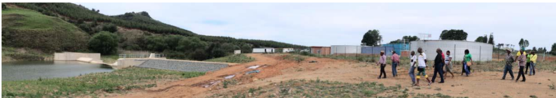
Figure 8.10 Weir and Package Plant on the Luhane River
