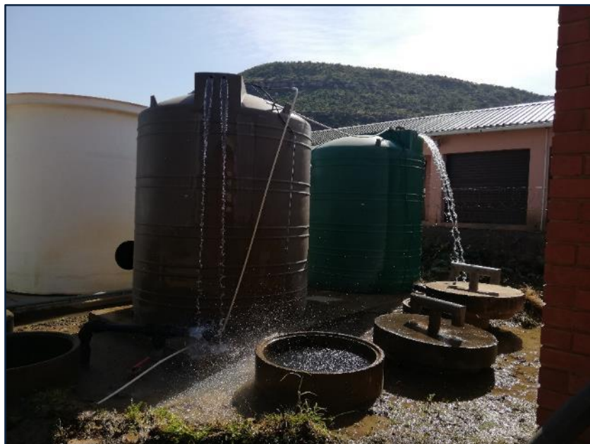
Figure 13.34 Tugela Estates WTP reservoirs (Umgeni Water 2019).
