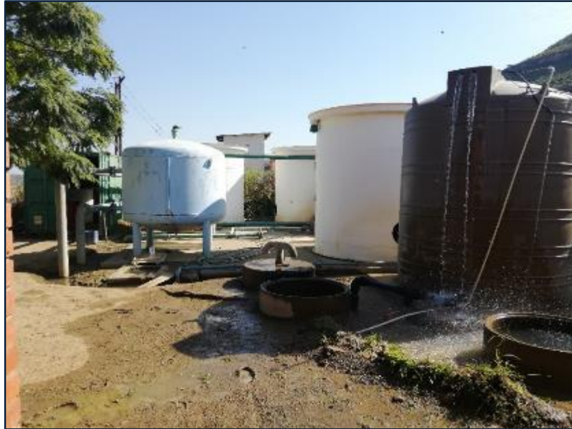
Figure 13.27 Tugela Estates Water Treatment Plant (Umgeni Water 2019).
