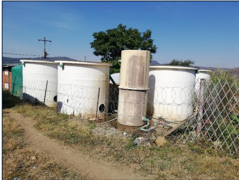
Figure 13.33 Tugela Estates WTP clarifiers (Umgeni Water 2019).
