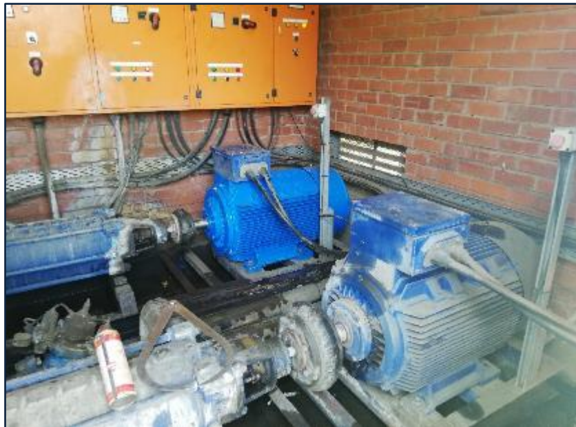
Figure 13.28 uMhlumayo Pump Station (Umgeni Water 2019).
