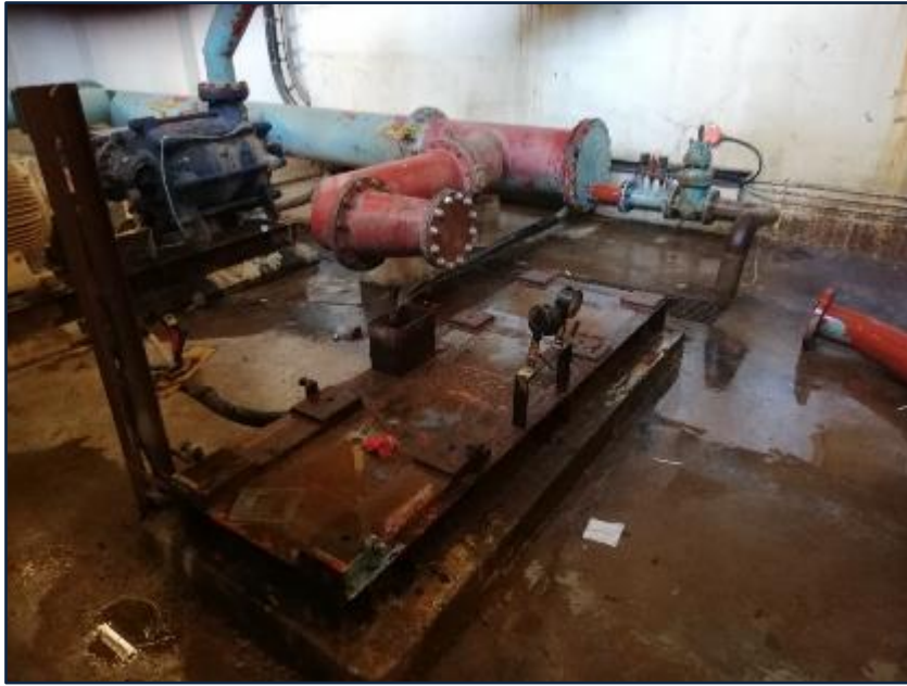
Figure 13.46 Petronella pump as of May 2019 (Umgeni Water 2019).
