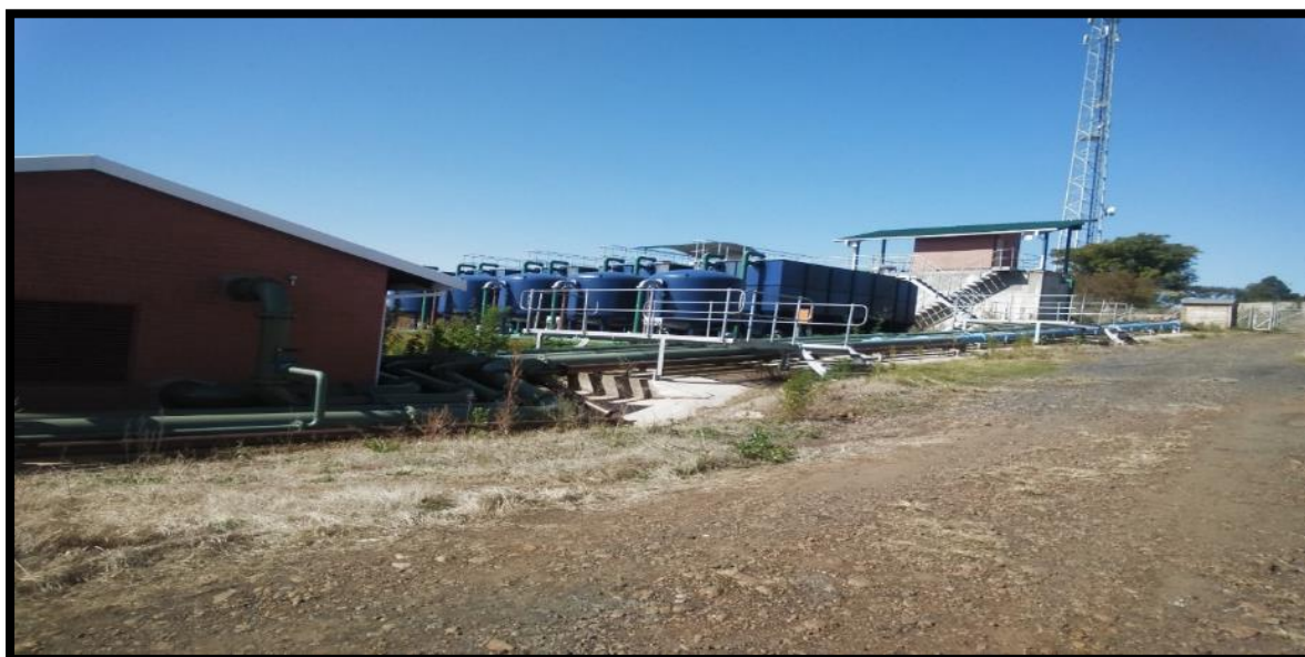
Figure 14.34 Photo of Durnacol Water Treatment Plant (May 2020).
