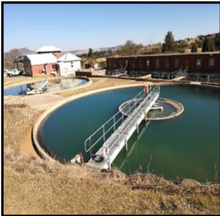
Figure 14.24 Photo of Biggarsberg WTP, Clarifiers (July 2019)
