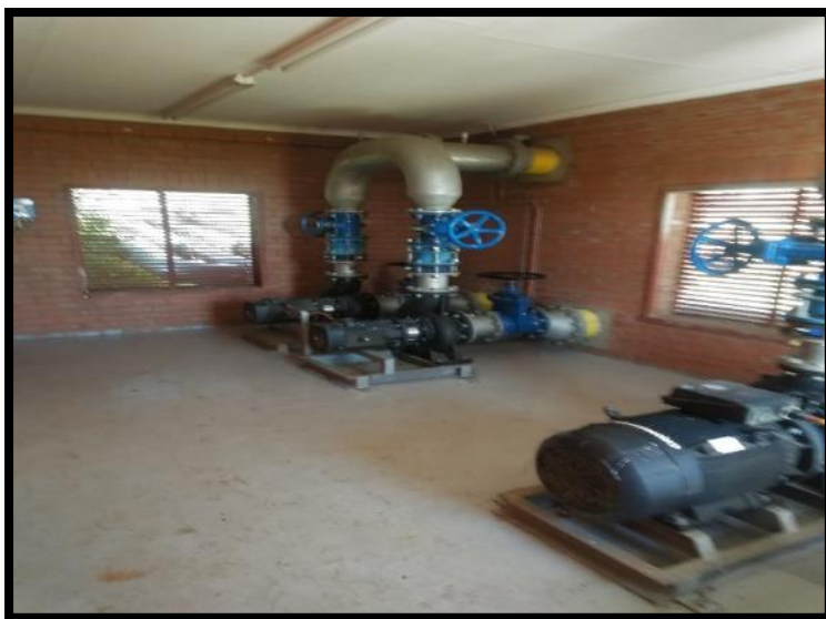
Figure 14.37 Durnacol Clear Water Pump Station (May 2020)
