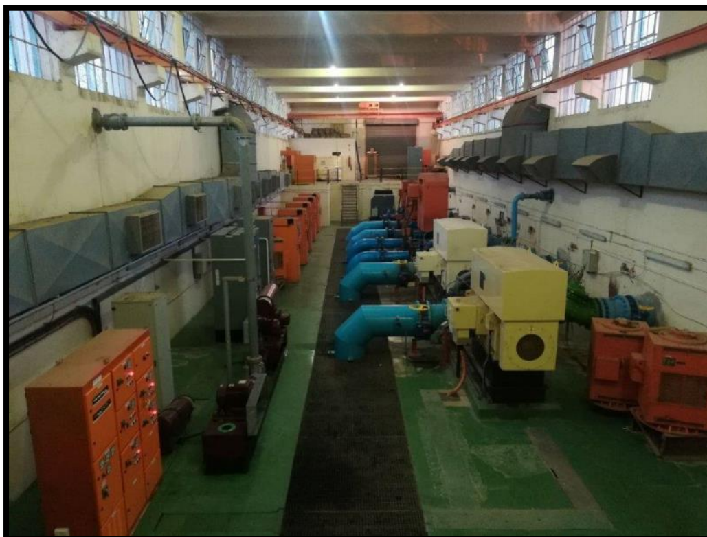
Figure 14.23 Photo of High Lift Pump Station at Ngagane WTP (May 2020)
