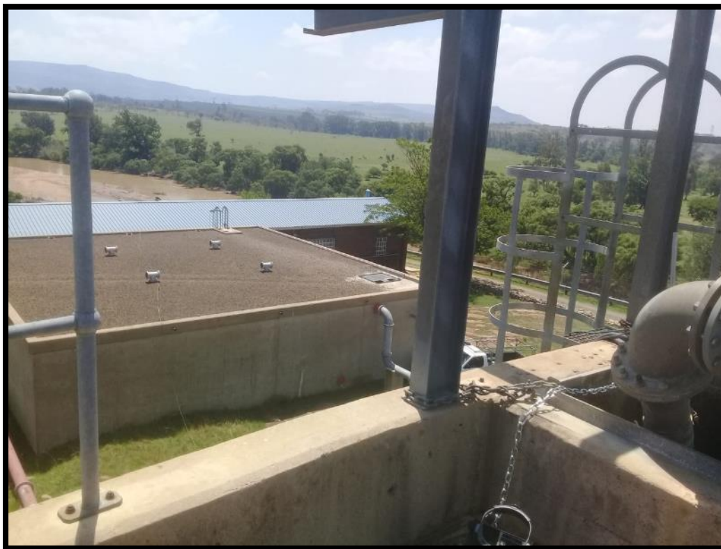
Figure 14.28 Photo of Vants Drift WTP (March 2020)
