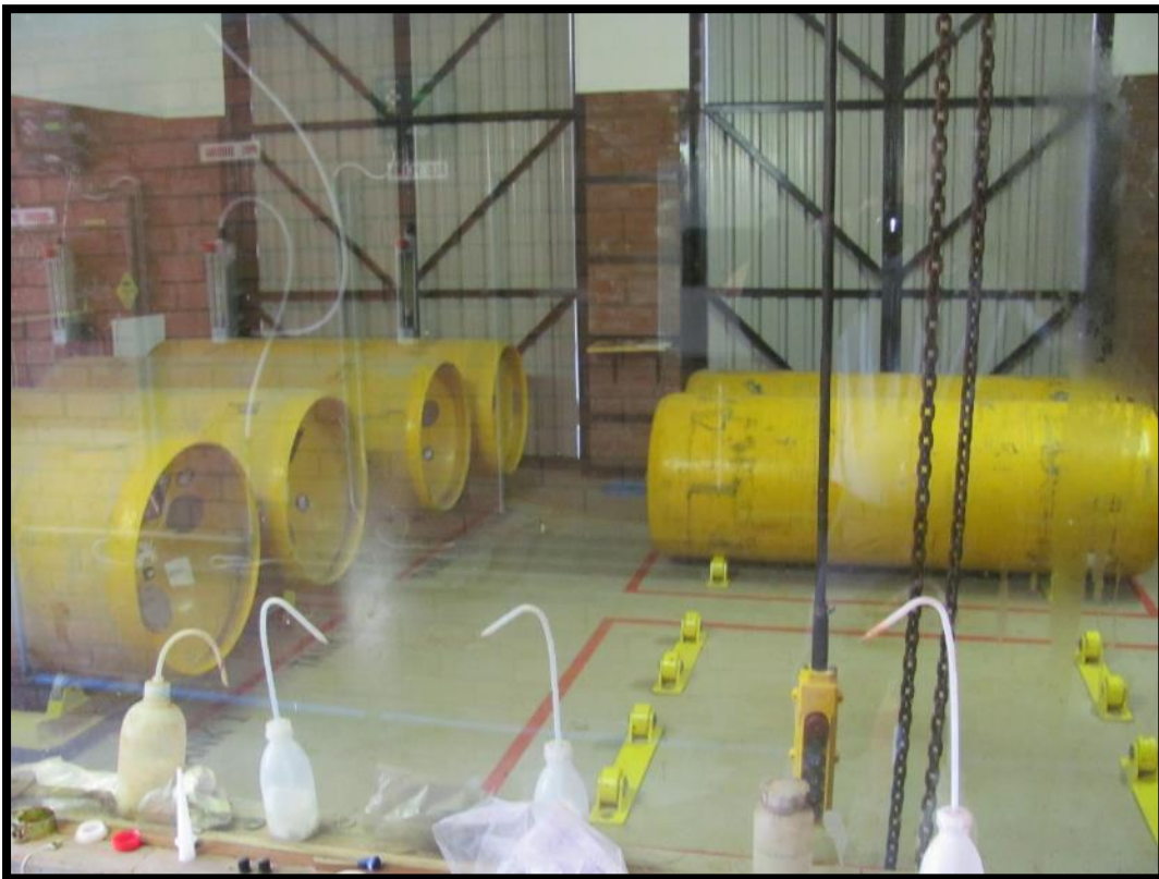
Figure 14.25 Photo of Chlorine Dosing Point at Biggarsberg WTP (July 2019)
