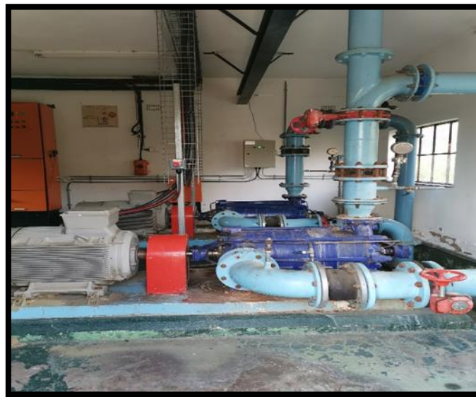
Figure 14.41 Utrecht Clear Water Pump Station
