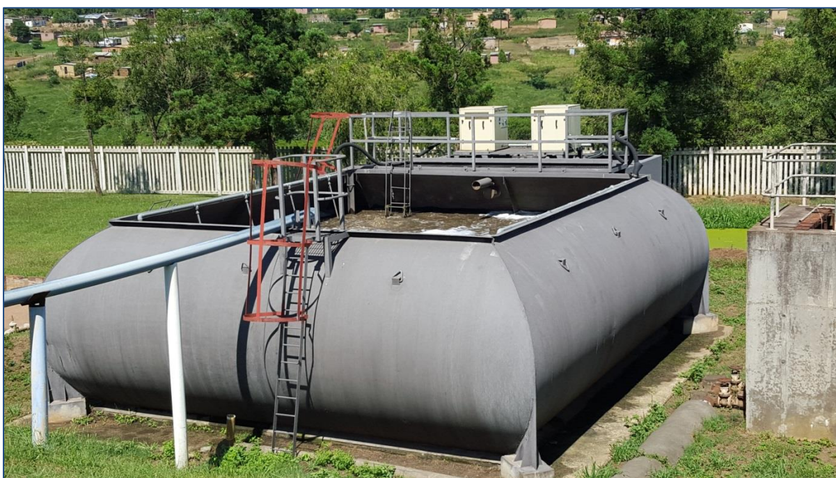
Figure 19.12 Sequencing Batch Reactor (SBR) Albert Falls North WWW.
