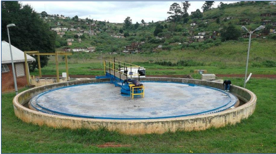
Figure 19.9 Clarifier No. 1 Ixopo WWW.
