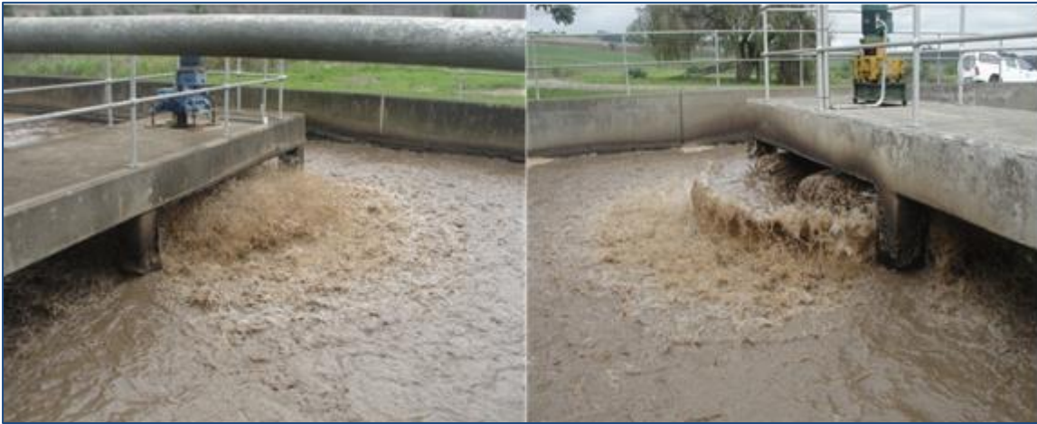
Figure 19.31 Different Mechanical Surface Aerators in Cool Air Reactor 1 and 2.
