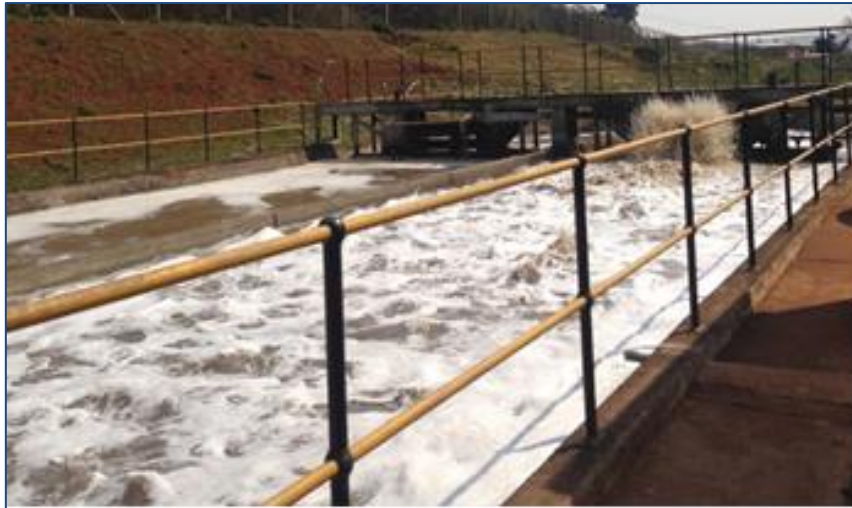
Figure 19.28 Appelsbosch WWT Oxidation Ditch (Aeration Tank).
