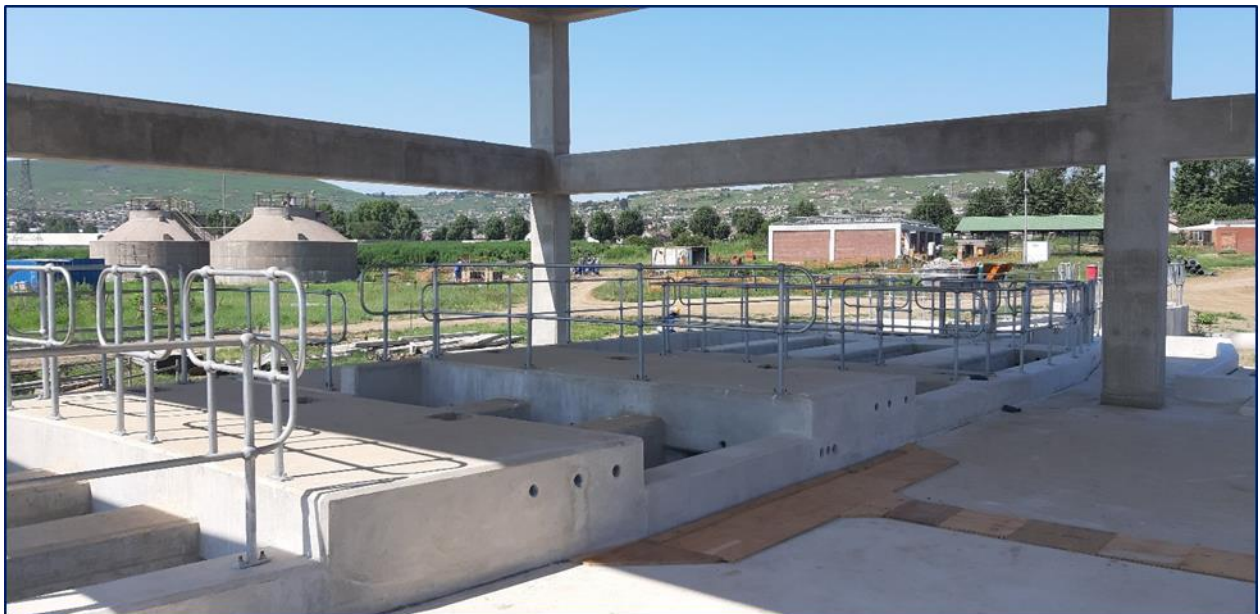
Figure 19.45: Mpophomeni Wastewater Works New Head of Works
