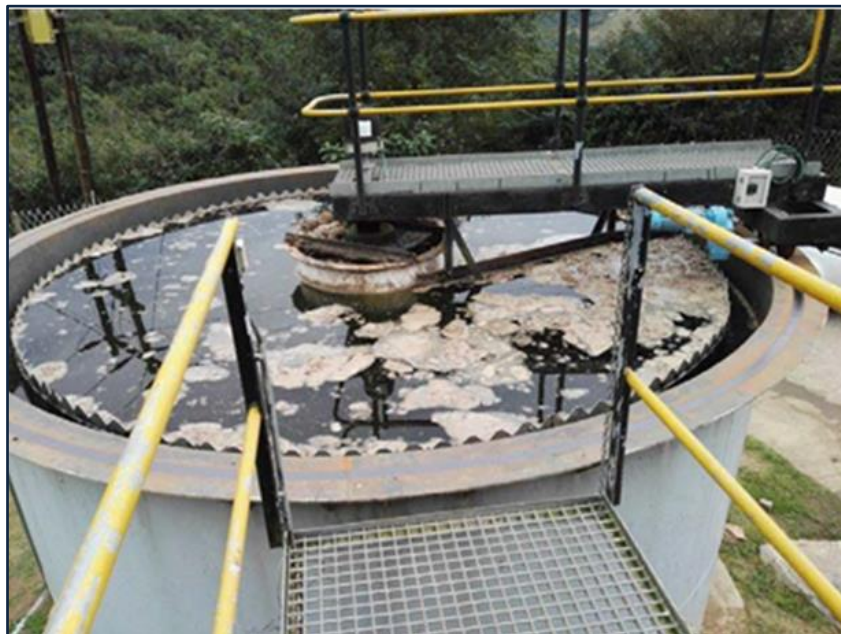
Figure 19.36 Camperdown Clarifier No. 2.
