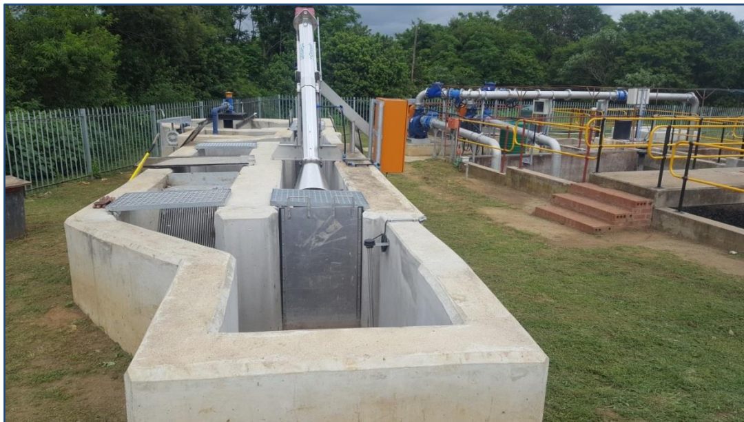
Figure 19.21 Lynnfield Park WWW head of works showing manual and mechanical screening channels.
