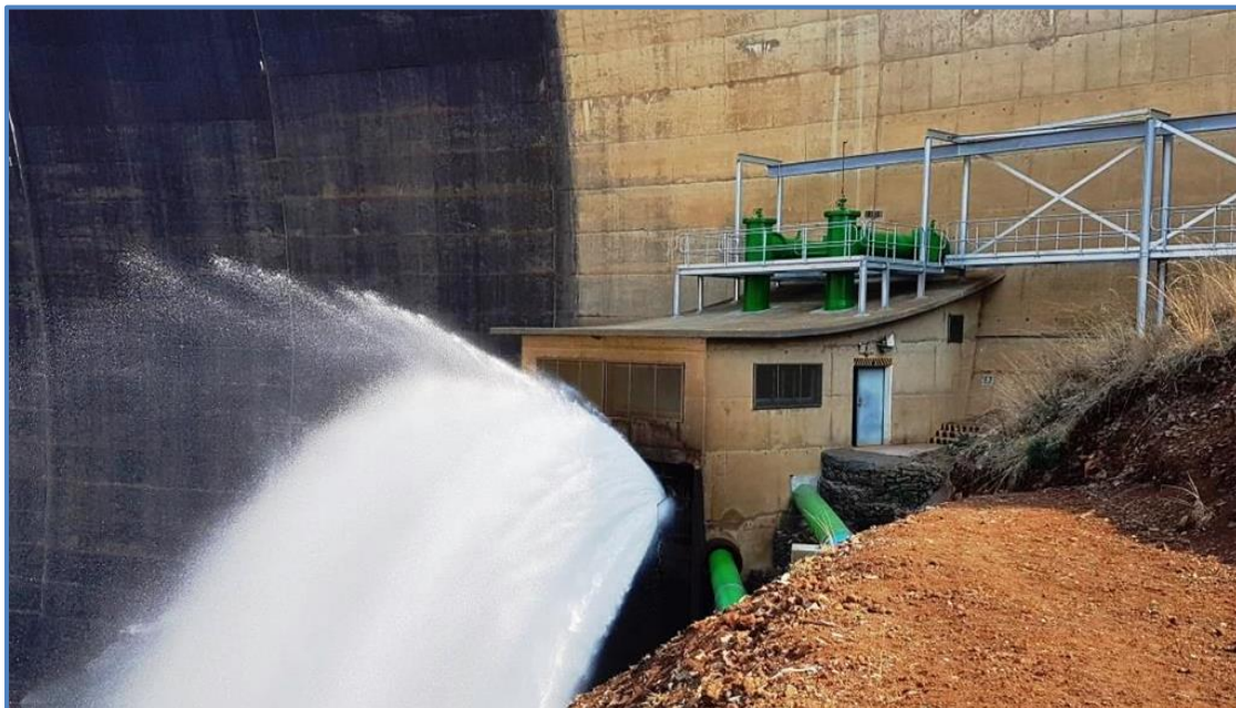
Figure 12.53 Abstraction point (Craigie Burn Dam)
